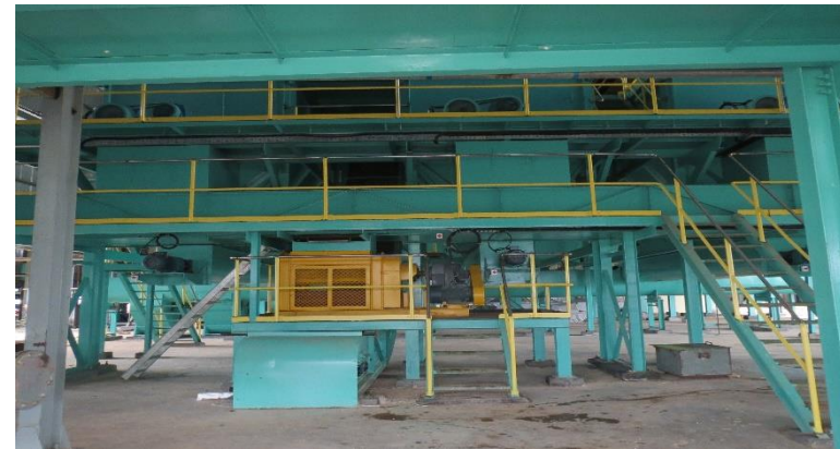
Thresher & Empty bunch Crusher
