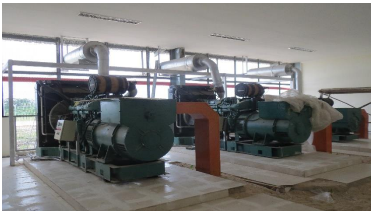
Engine Generator Set
