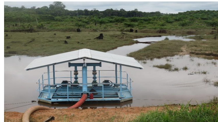
Raw water intake pump
